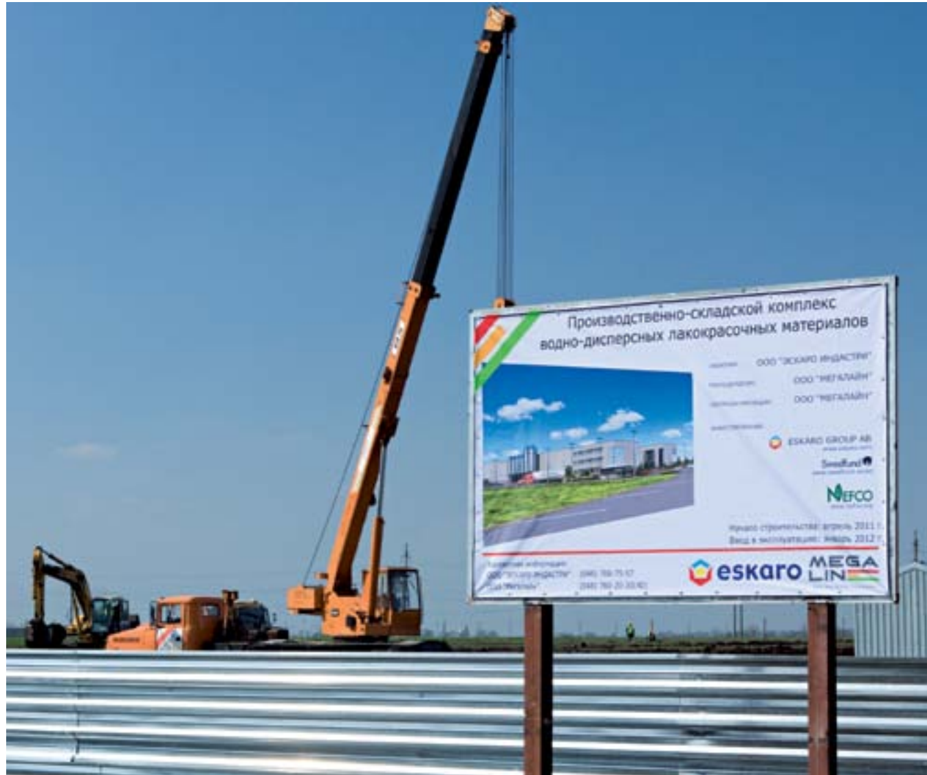
The Eskaro construction site in Odessa in April 2011. The new factory will utilise closed circuit production techniques.
