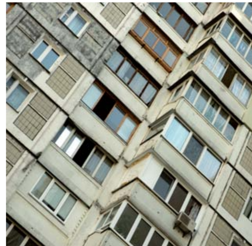
Block of flats in Kiev. The E5P will promote modernisation of district heating systems in Ukraine.
